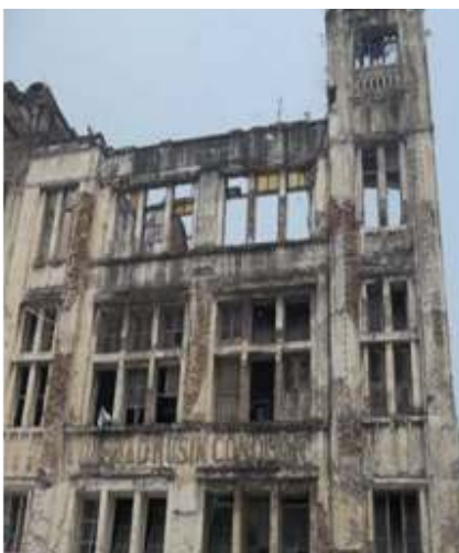
Weathering of building walls
